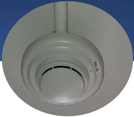
Typical Suite Smoke Detector
